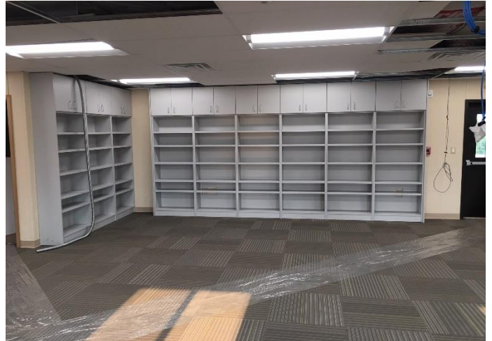
Library bookcases are in and all carpet installation is complete.
