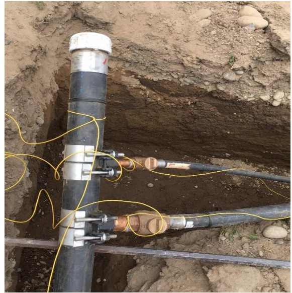
The installation of the new 3" water main passed the pressure test at 150lbs for 2 hours.
