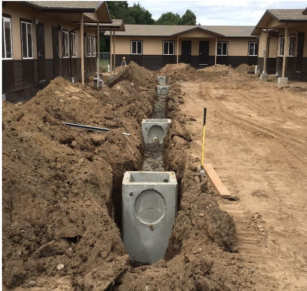
The final infiltration trench for the down spout drains on the interior of the campus is just being completed.
