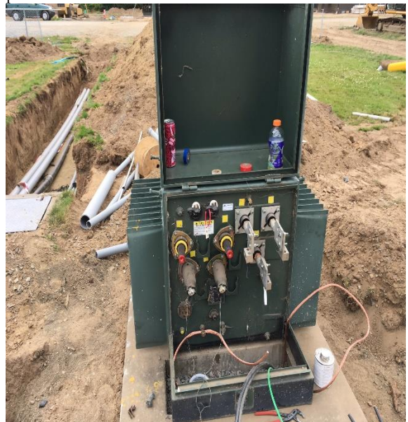
Transformer connections have been made and power will be energized to the portables next week.
