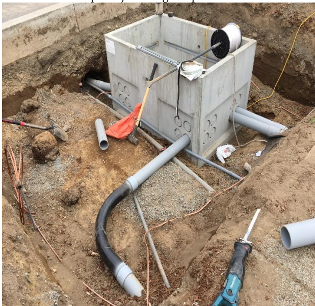
The second of two new underground electrical vaults were installed this week.
